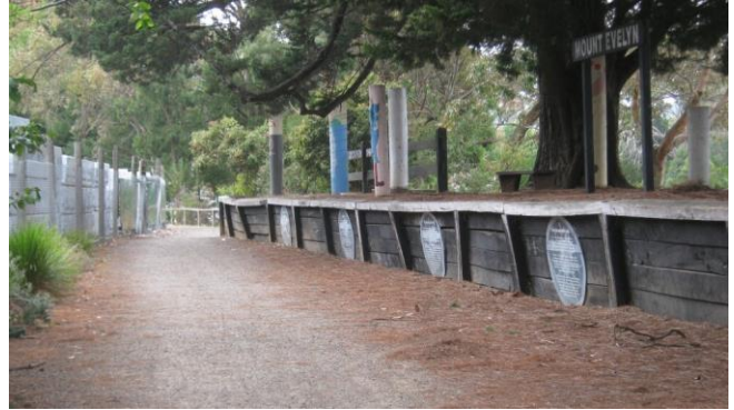
Station platform with leaning wall and trail bottleneck at the far end. Photo Kevin Phillips.
